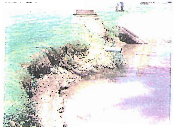
Photo 2: Erosion at outlet of the concrete channel
