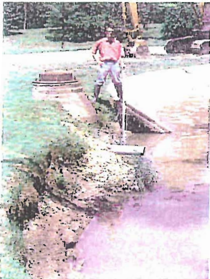
Photo 7: Erosion at end of concrete channel
