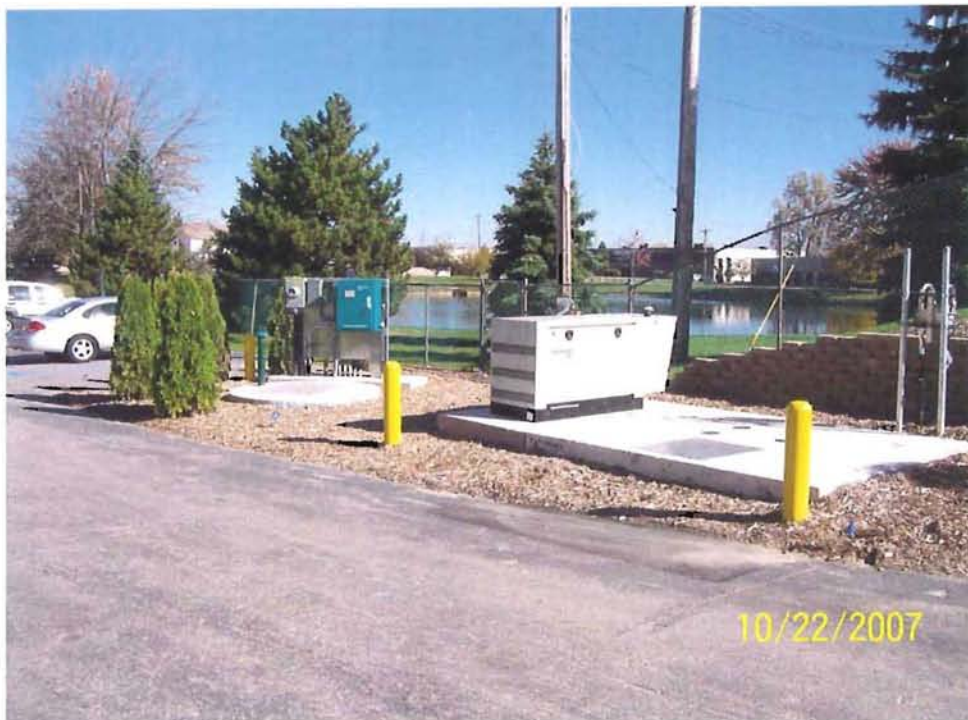
Stonehenge Lift Station
