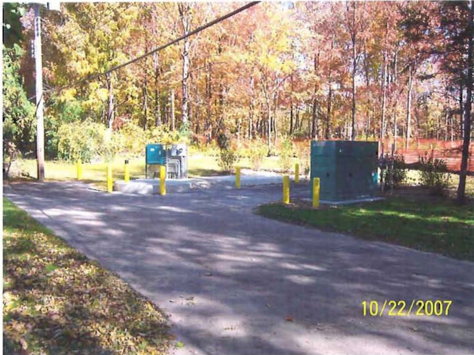
Country Place Lift Station
