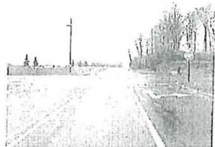
Existing intersection looking east shows deficiencies in geometrics and lane continuity.
