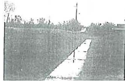
Draining west, existing paved ditch adds to steep slope issues upon road widening.
