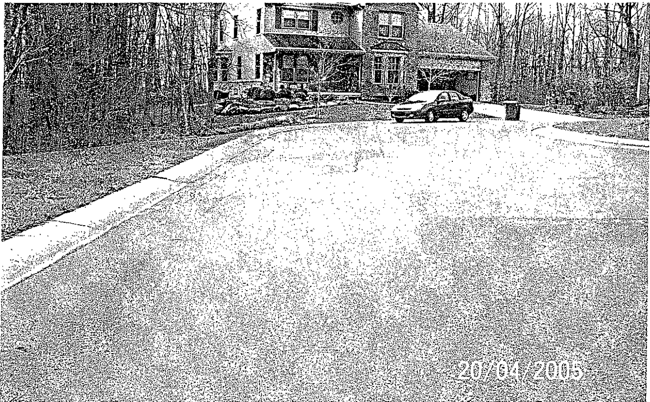
Stonewall Ct. Variety of surface cracking.
