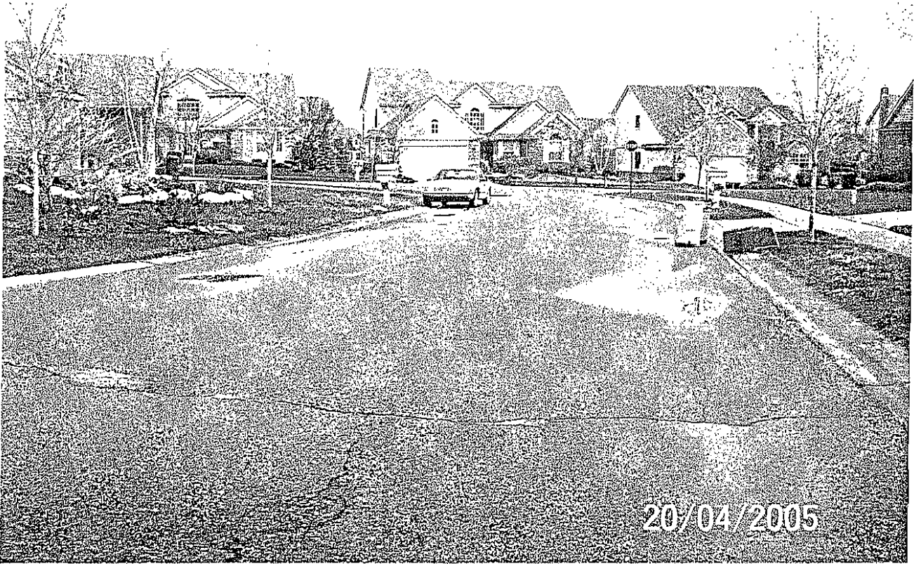
Stonewall Ct. at cul-de-sac island, looking toward Sandstone Cracking and multiple areas of surface ponding.
