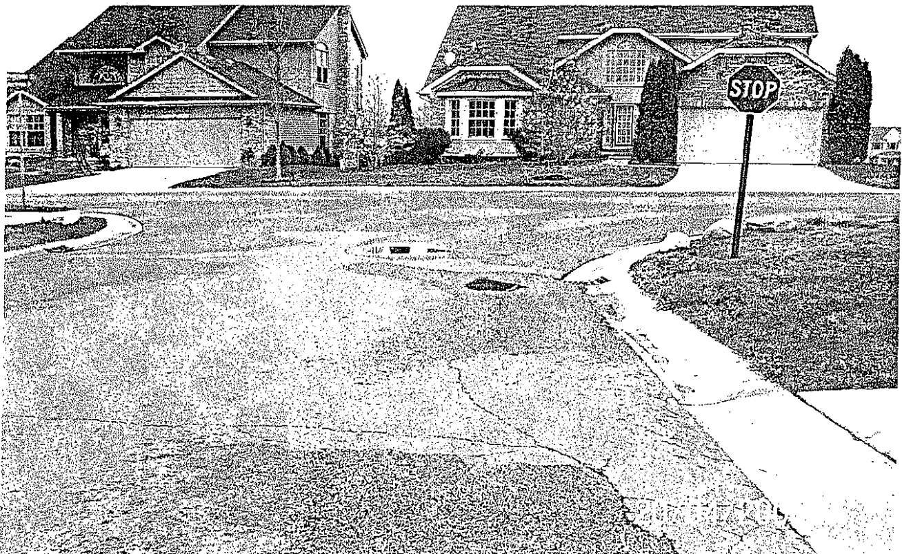
Brookstone at Hearthstone Low point and ponding in front of catch basin with transverse cracking.
