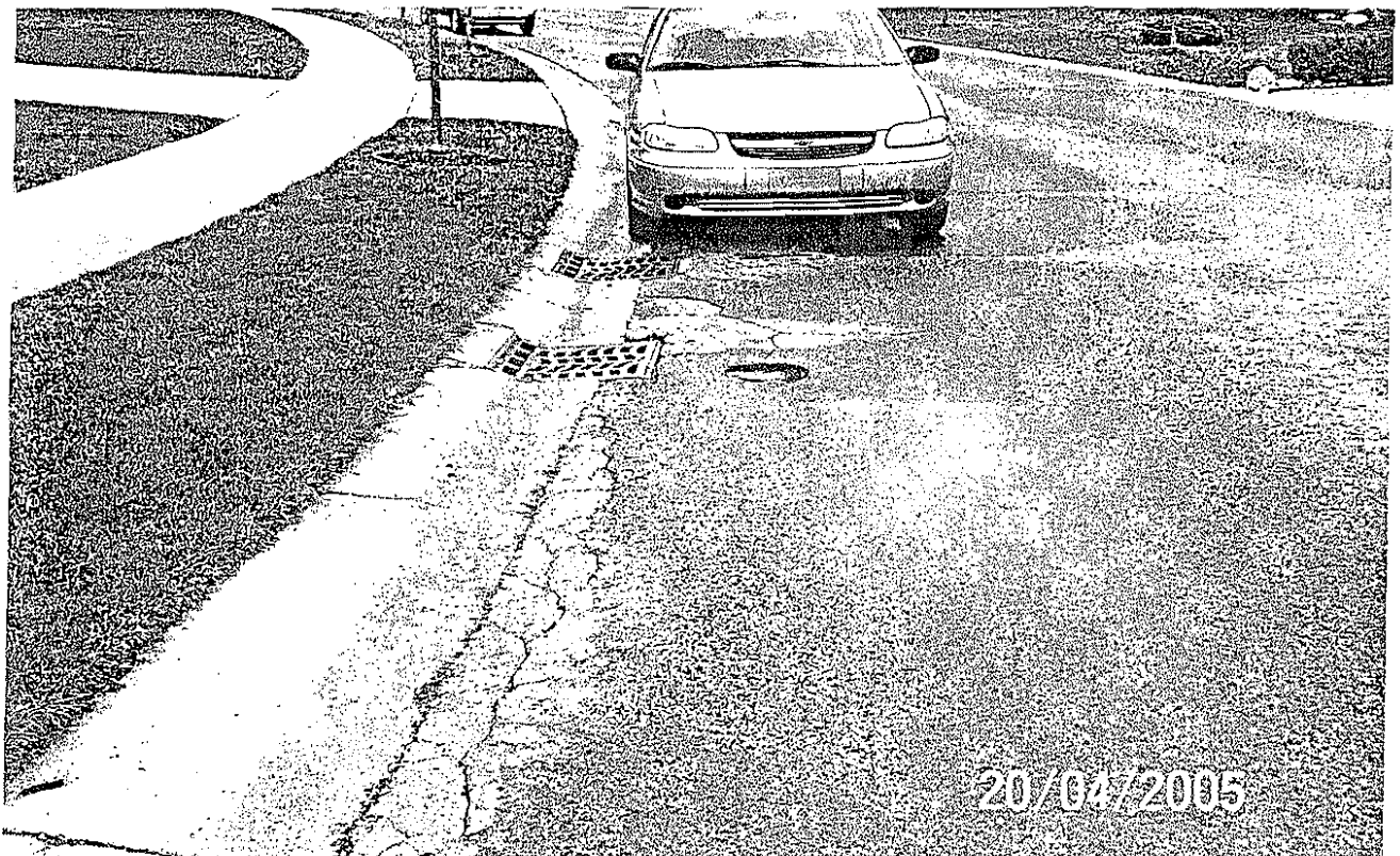
Brookstone at house no. 42813 Minor ponding in front of catch basins and cracks at edge of metal.
