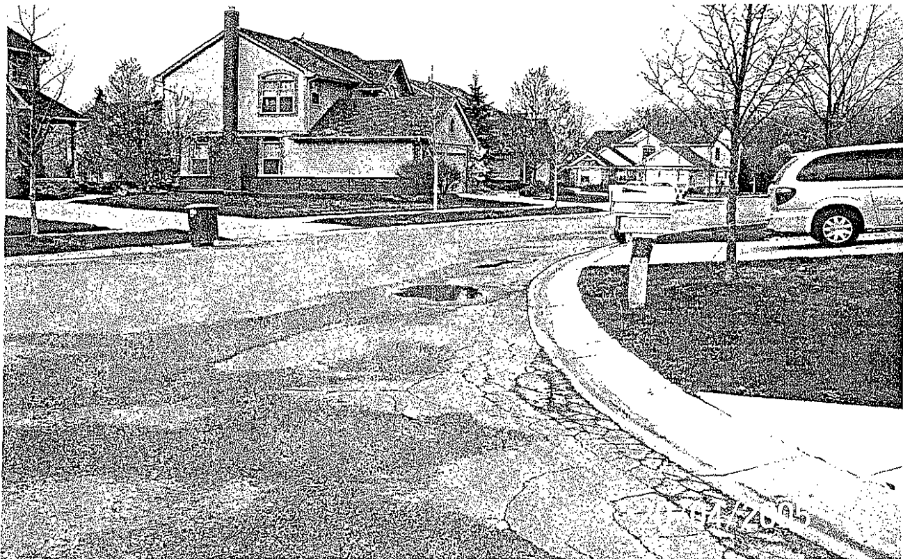
Ledgeview on north side of road at cul-de-sac curb return Low points in pavement surface with ponding and edge cracking.
