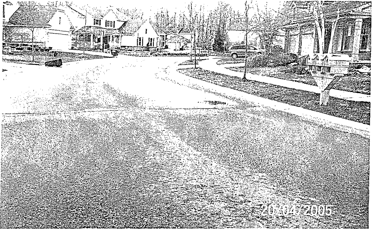
Brookstone between house no. 42769 and house no. 42797 Low point in pavement surface and transverse crack.
