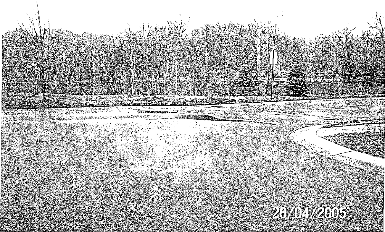
Sandstone west of Hearthstone Heaved pavement is causing storm water to pond on street surface
