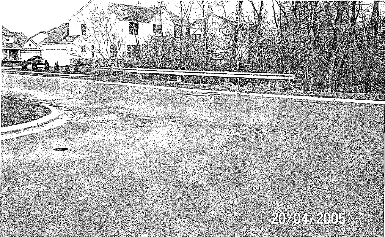
End of Sandstone at eyebrow cul-de-sac Low point on pavement with ponding upstream of catch basin. The crack runs across the length of the intersection.
