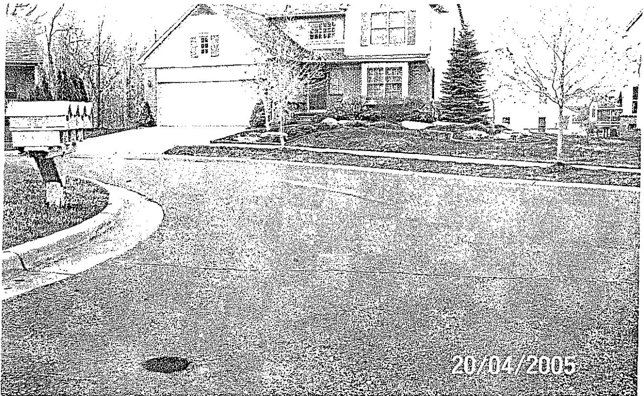
Quarry Ct. at north side of cul-de-sac island Londitudinal and transverse cracking.
