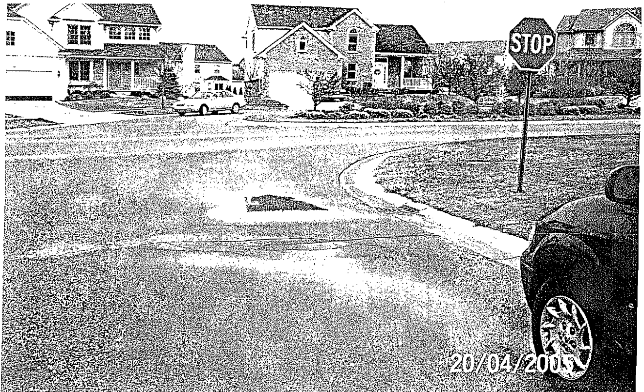
Quarry Ct. at Sandstone Ponding and cracking in front of catch basin.
