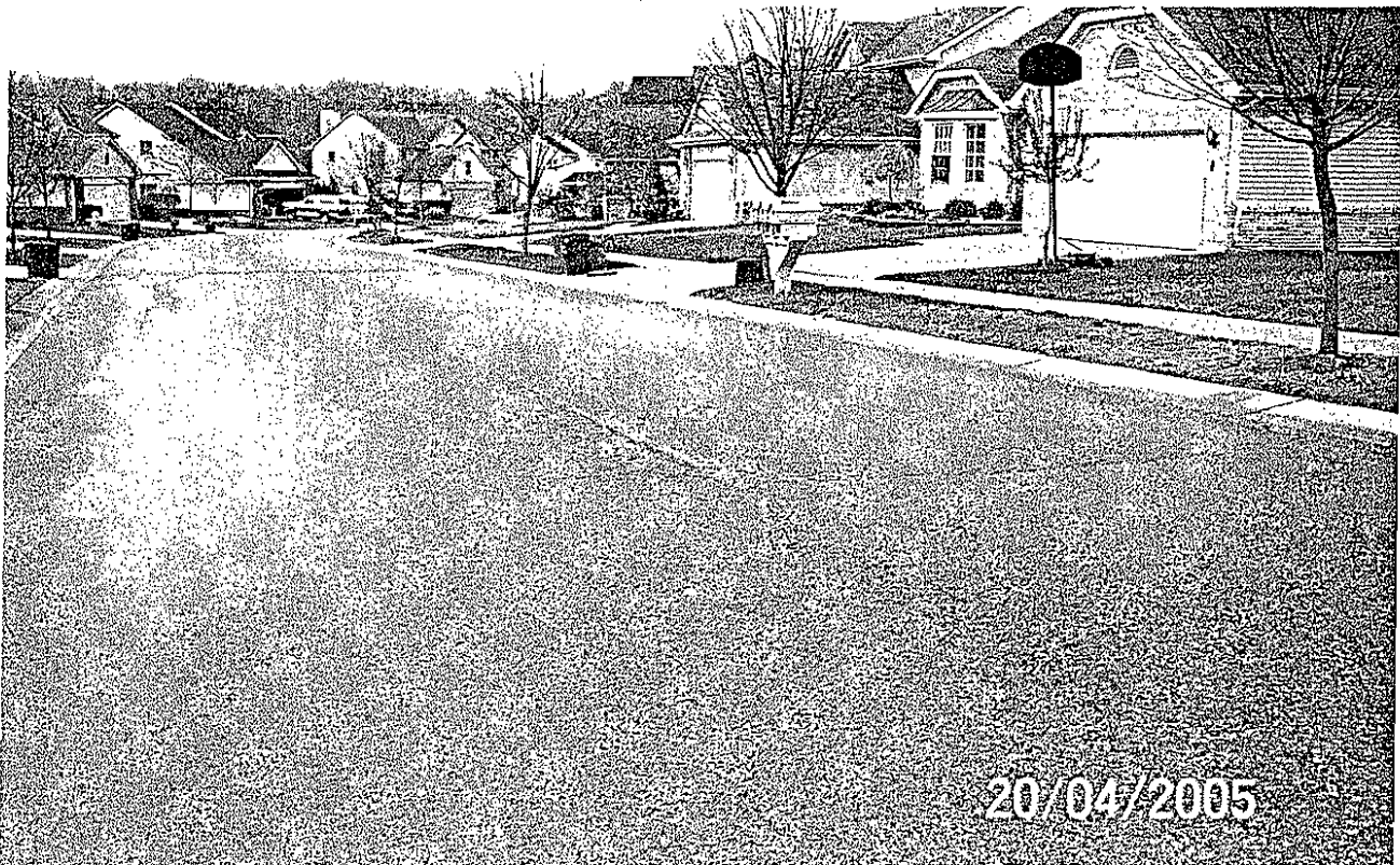
Sandstone at house no. 43094 Transverse and longitudinal cracking.
