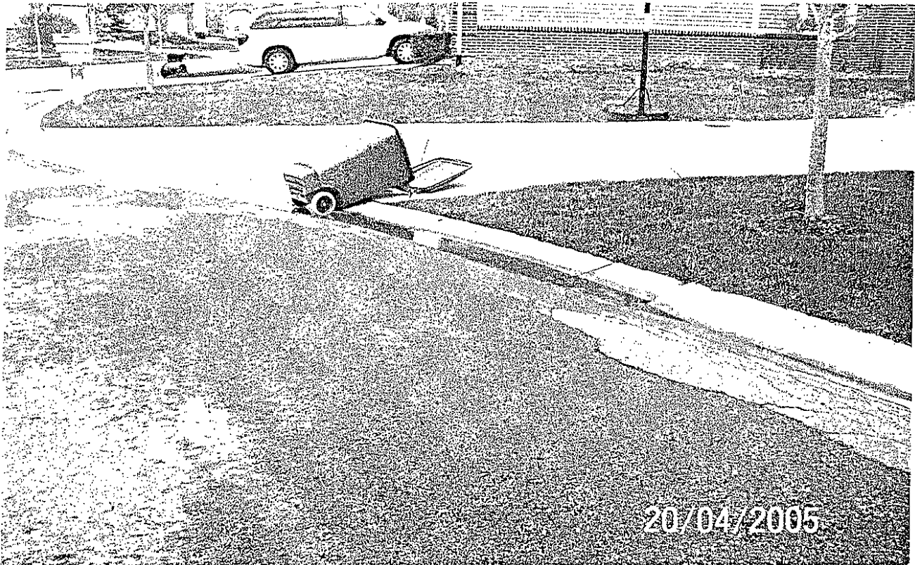
Ledgeview at house no. 42790 Pronounced low point in curb with ponding and edge cracking.
