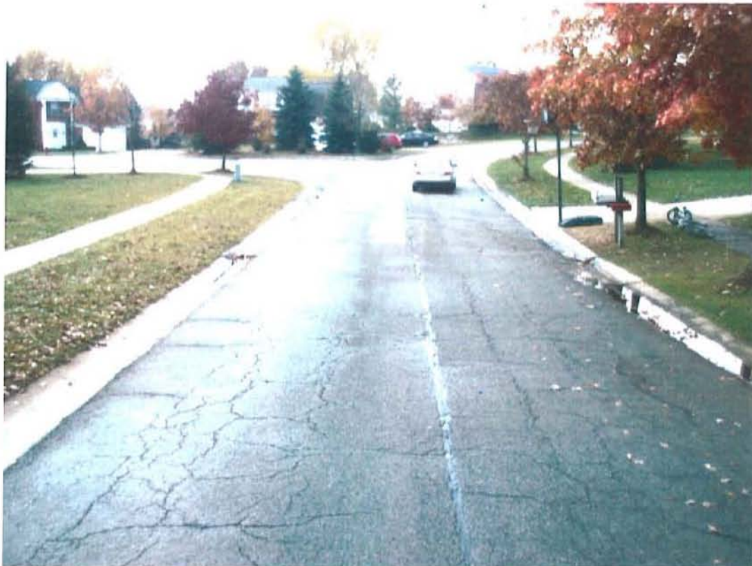
Asphalt street still structurally sound, but contains many cracks in the wheel path. Candidate for thin asphalt overlay.
