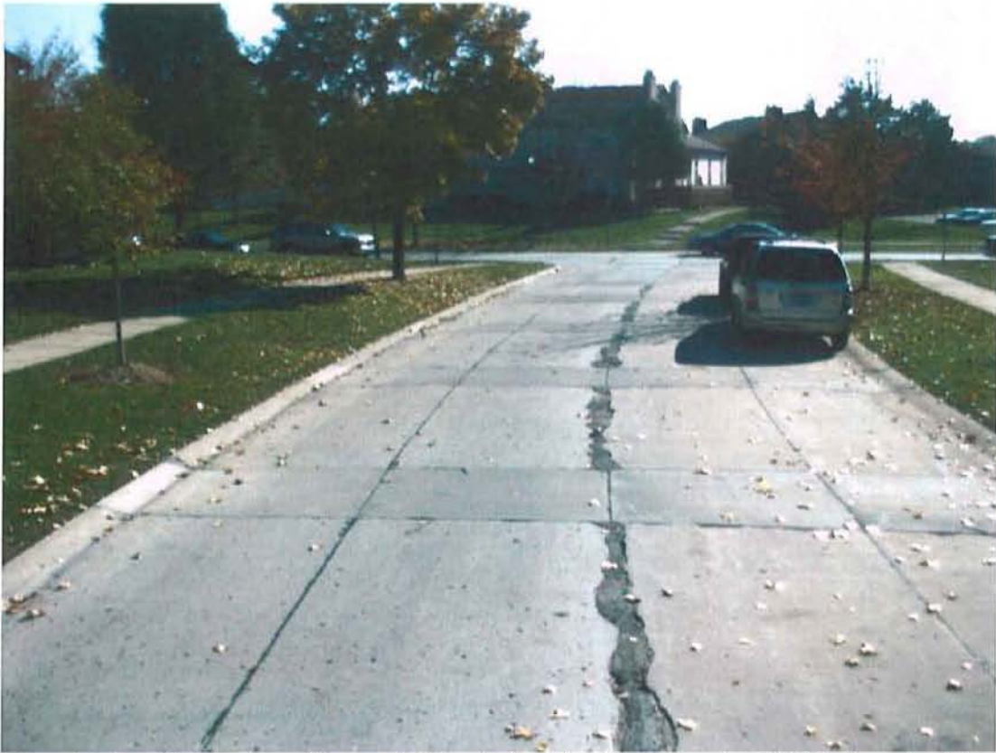
Concrete street in good condition containing bad center joint. Repair of joint is important to prevent further deterioration of adjacent concrete slabs.
