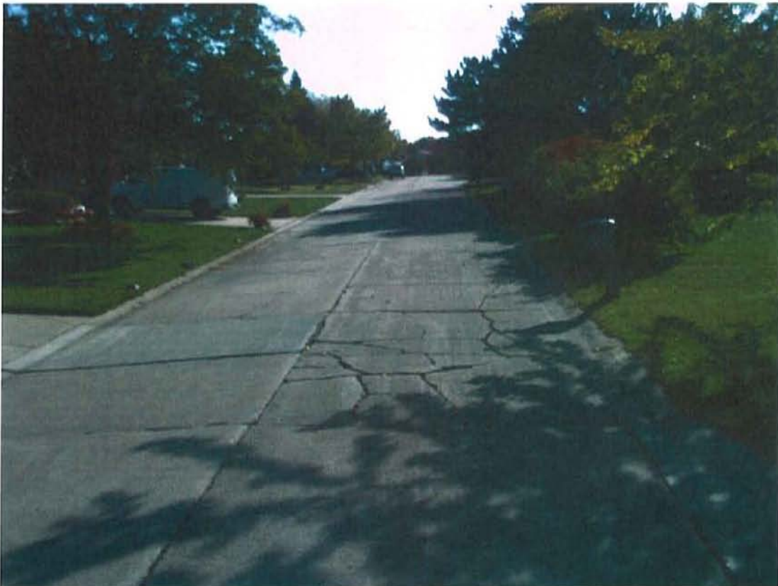
Concrete street in generally good condition with discrete failure. Candidate for discrete partial-depth or full-depth repair.
