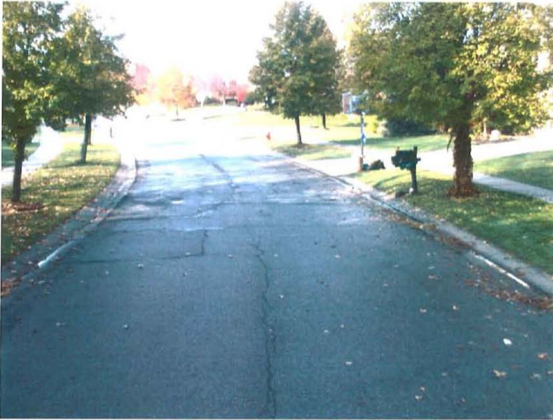
Asphalt street in generally good condition with small area of failure. Candidate for discrete partial-depth or full-depth repair.
