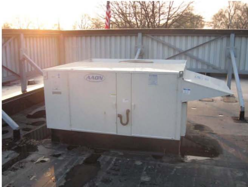
Photograph No. 2 Electric heat pump rooftop unit. Electricity consumption should be monitored for winter months.
