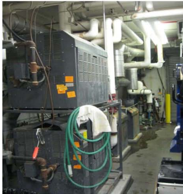
Photograph No. 4 Traditional Boiler System for ice arena. Requires purchase of natural gas.
