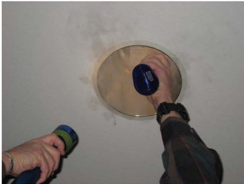
Photograph No.6 All of the can lights are connected through ceiling ventilation to outside air. Smoke puffed into recessed can descends rapidly due to cold air current. Replace leaky baffles with air tight baffles.
