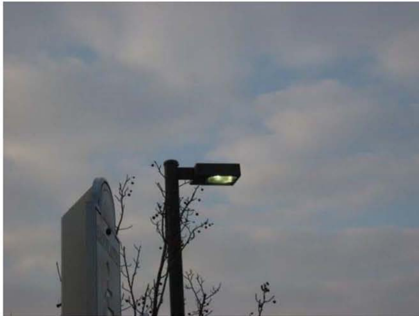
Photograph No. 1 Parking lot lights on when it is still daylight. Check photo sensors.
