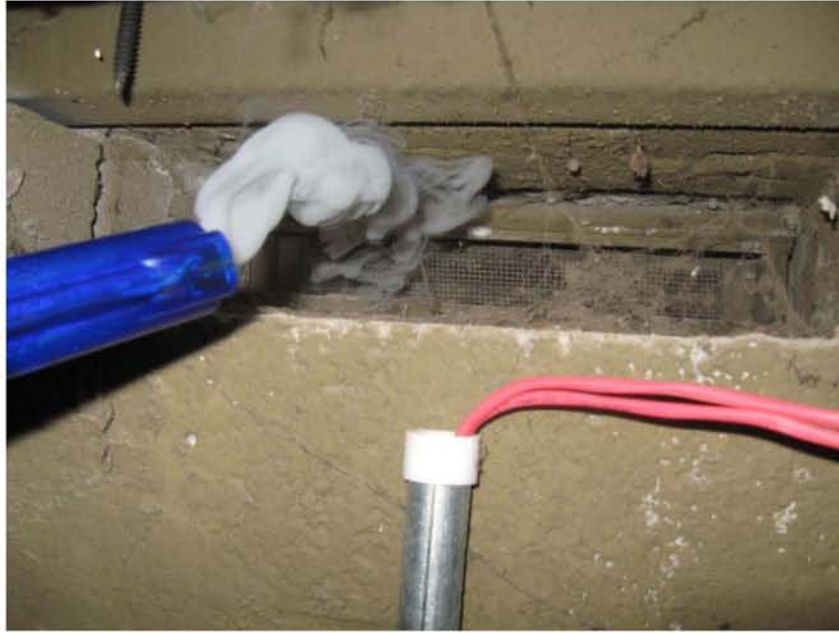
Photograph No. 1 Smoke rapidly leaving the mechanical room through a vent hole that is no longer necessary.
