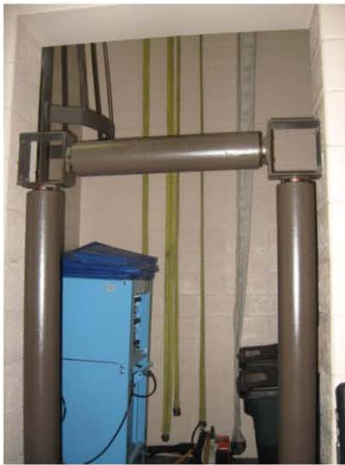
Photograph No. 3 The opening to the hose drying tower, directly connected to the heated equipment bay.
