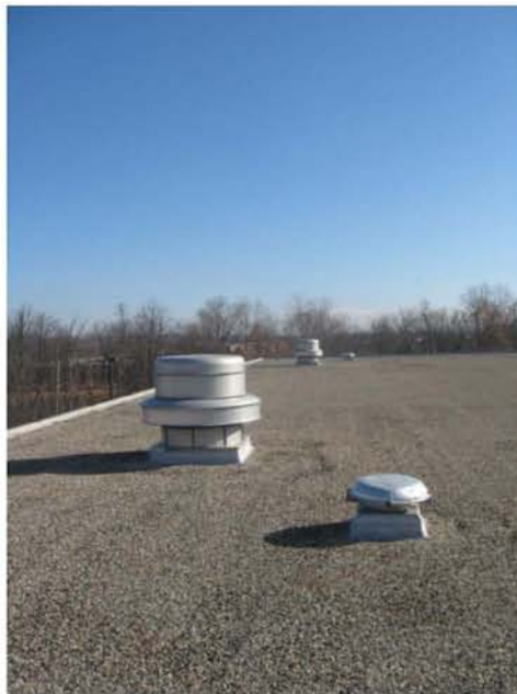
Photograph No. 4 Rooftop mushroom fan for ventilation system
