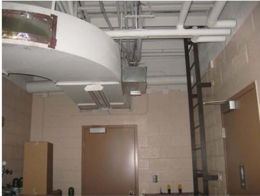
Photograph No. 5 Boot on HVAC trunk line forces conditioned air down the corridor into the equipment bay and out of the building through the hose drying tower in the summer and the winter.
