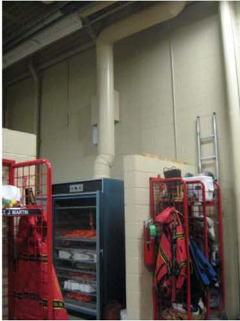
Photograph No. 3 Hose drying machine is an advantage over open chimney in fire house.
