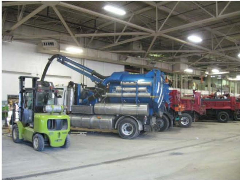
Photograph No. 2 View of ventilation and HVAC ductwork.
