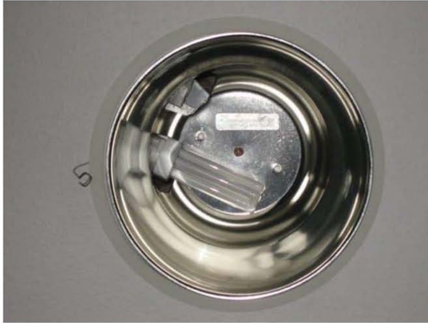
Photograph No. 5 Recessed Can lights are not air tight.
