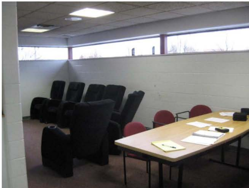
Photograph No. 6 Un-insulated block walls and substantial glazed area – typical of fire house construction.
