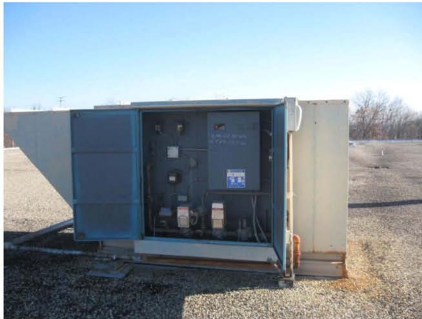
Photograph No. 8 Direct fired system is legal only if 100% fresh air is used. All take dampers on this unit are closed. The linkage to the actuator is disconnected. Control of damper needs to be reestablished.
