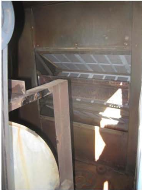
Photograph No. 7 Makeup air unit is direct field system. All products of combustion enter the occupied space.
