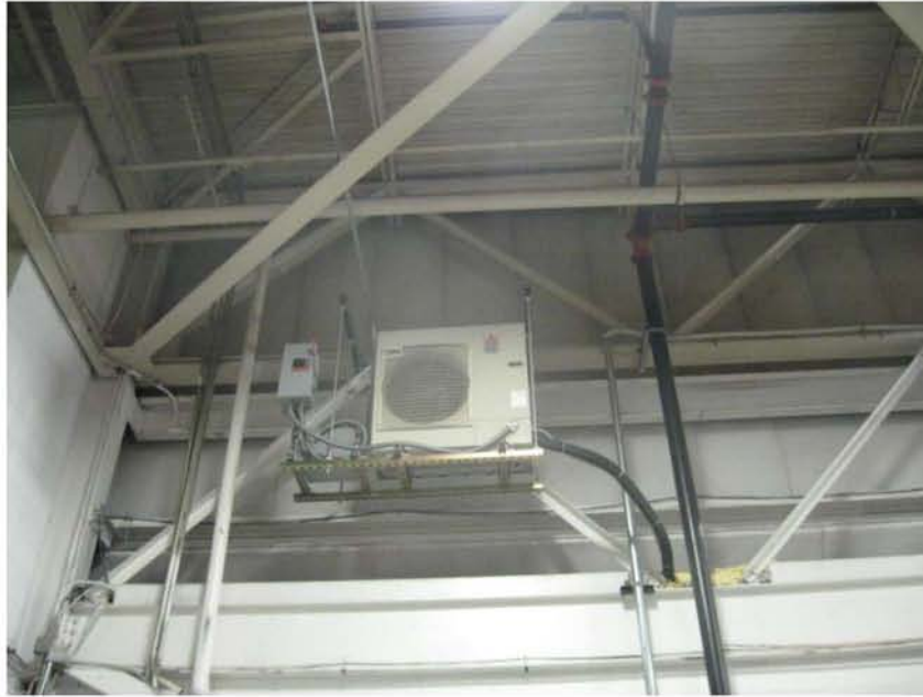
Photograph No.11 Drip pan and drain to outside needed below condenser.
