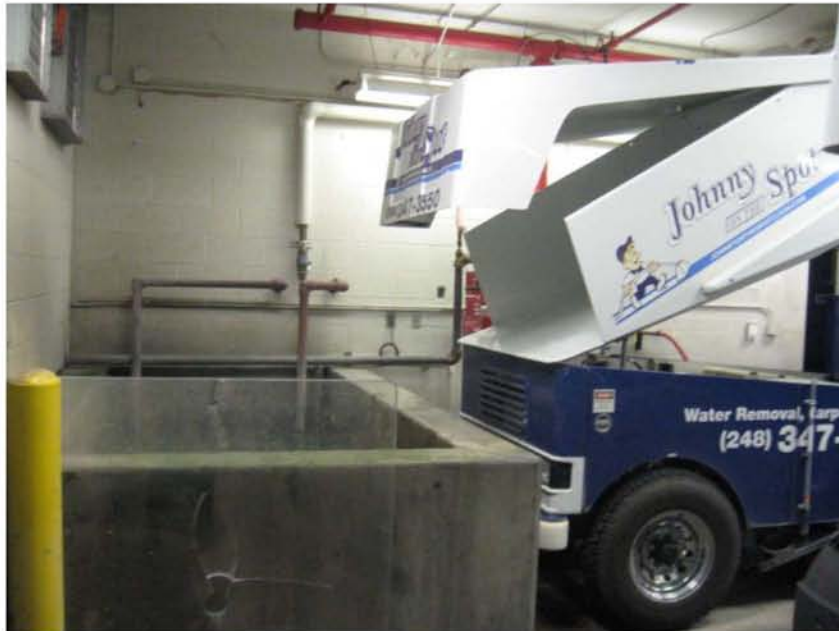
Photograph No. 2 Pipes for hot gas snow melting system are too small, forcing high head pressure. Replace with properly sized stainless steel piping.
