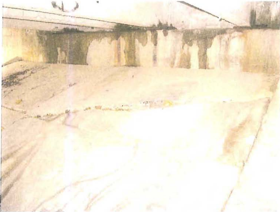
North Abut. Seat below beams 3W-6W wet. Beam seat is spalled between beams with exposed rebar. Spalls extend under bearing areas approx. 5%.
