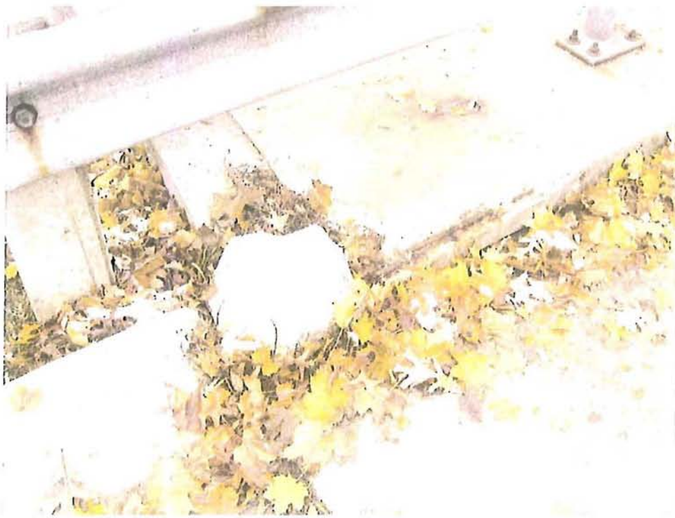
Toe of west sidewalk and top of abutment wall – spalled concrete with exposed reinforcement.
