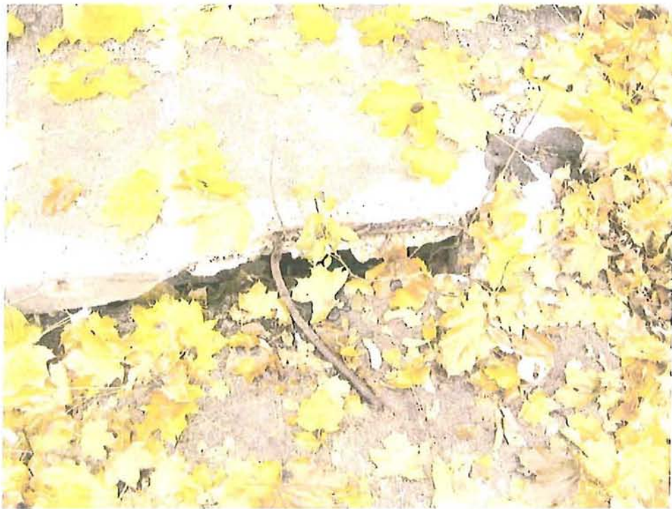
Toe of west sidewalk – spalled concrete, expose and corroded reinforcing steel.
