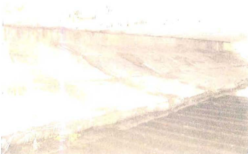
South abutment and slope protection. Slope paving is undermined, settled, and cracked throughout.
