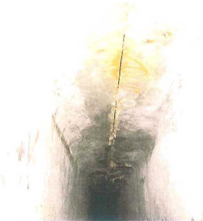
Typical condition of joints between beams – Top flange is wet with efflorescence and rust staining.
