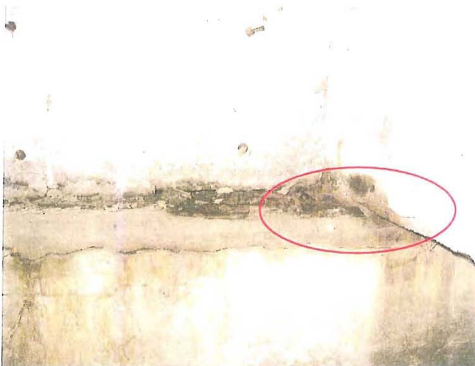
Typical condition of bearings. Bearings have heavy pack rust and section loss. Concrete at bottom of beam at bearings is cracked.
