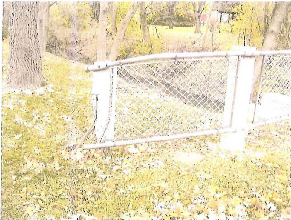
Damaged concrete post in the northeast quadrant of the bridge.
