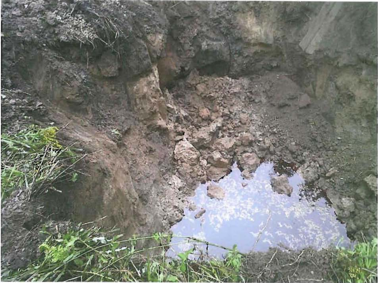
Leaking Heating Oil in Excavation
