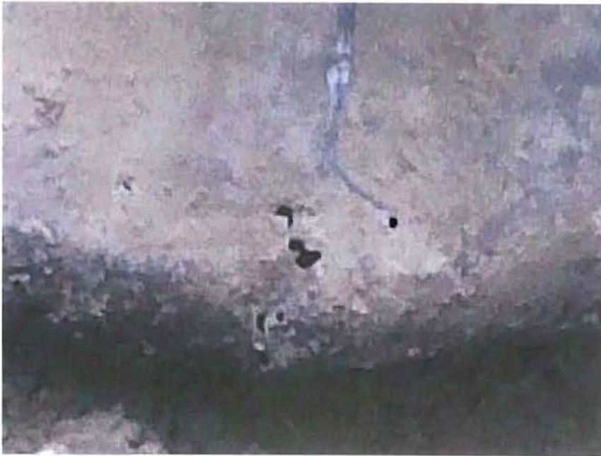
Corrosion perforations in tank
