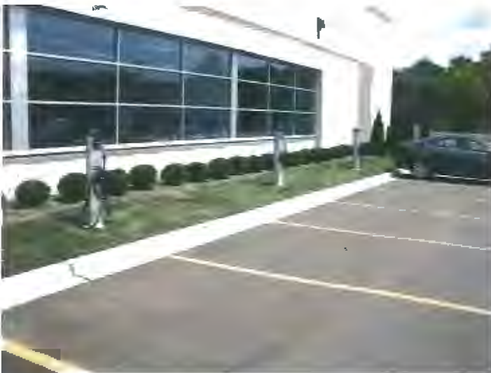
PEV Charging Stations and Spaces (Kistler North America, Novi)
