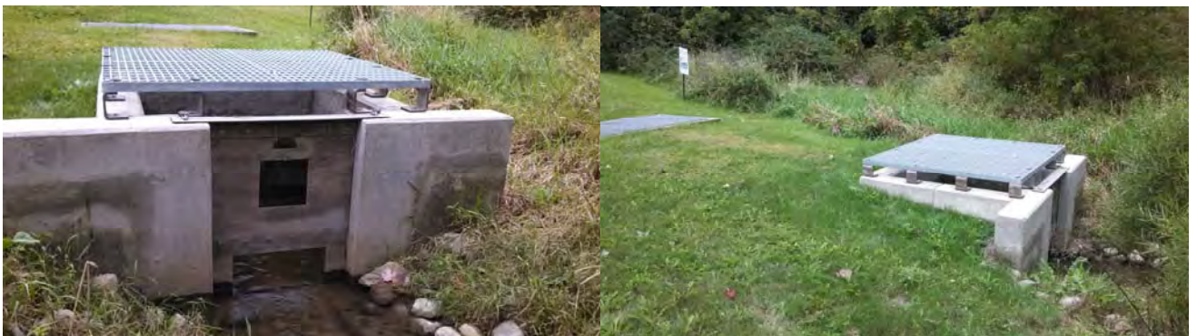
New outlet control for Lexington Green Regional Detention Basin
