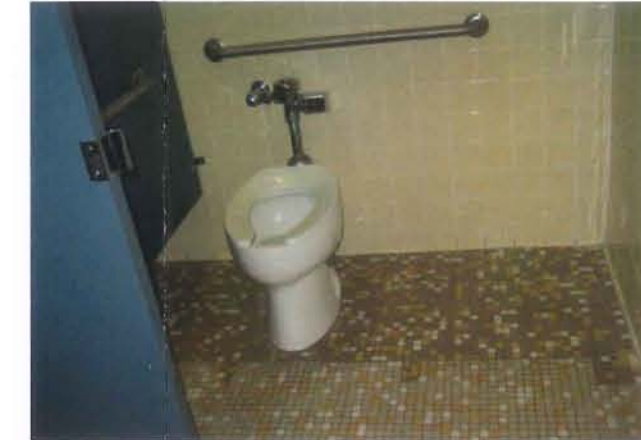
Bathroom floor patch, typical through out building.
