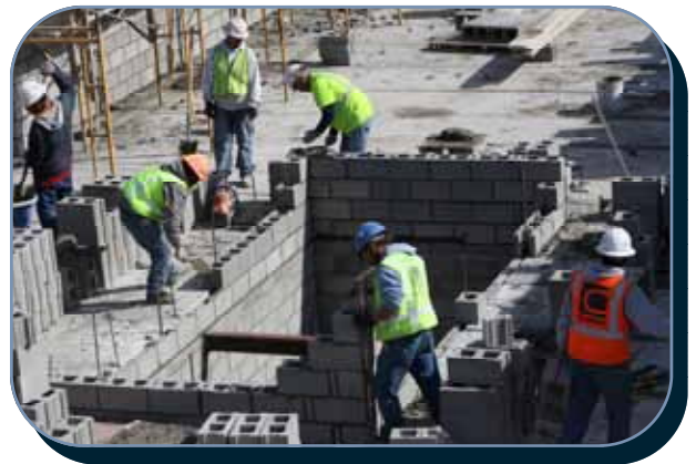
Construction crews work on the new Hyatt Place Hotel, scheduled to open in summer 2013 at the Suburban Collection Showplace.
