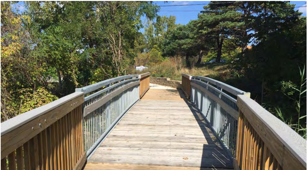
Pre-fabricated Bridge along Meadowbrook Road between Bridge Street and Grand River Avenue
