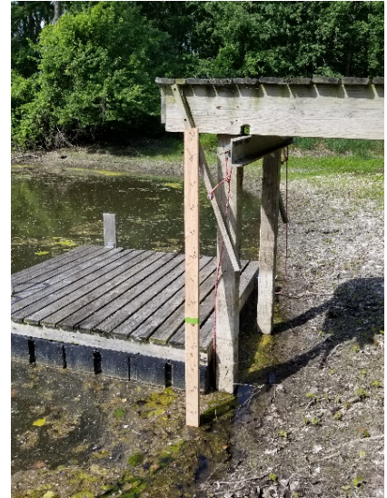
Water Level "gauge"
