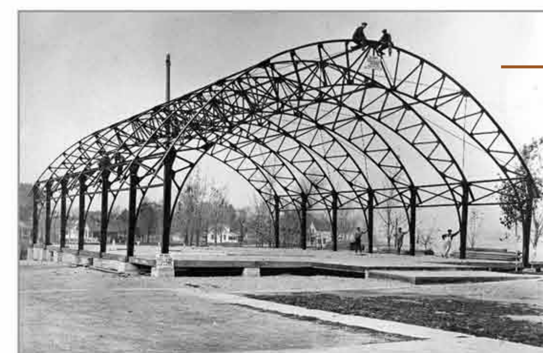
The casino under construction in 1924. Owner Louis Talletene joined a flurry of development of bath houses and dance pavilions at the lakeshore that began in 1919. Photo courtesy of the Novi Historical Commission.
