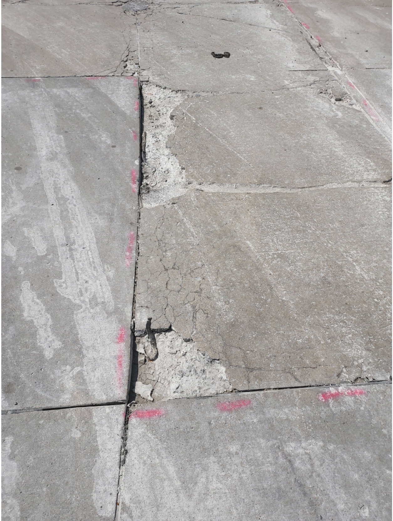
Existing concrete ASR condition of Highlands Drive in Meadowbrook Glens Subdivision as of 6/23/23.
