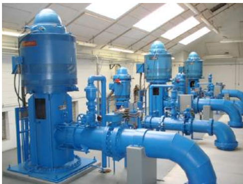
Pumps in the Celestial Road Pump Station
