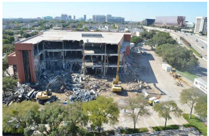
The former Sakowitz Department store, being demolished to make room for Whole Foods.
