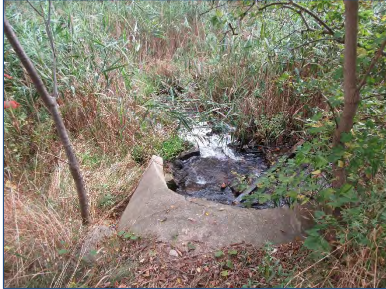
Photo 3. Stormwater inlet (Seeley Drain) located along the western property boundary in the southwest section of the site (ECT, October 10, 2017).
