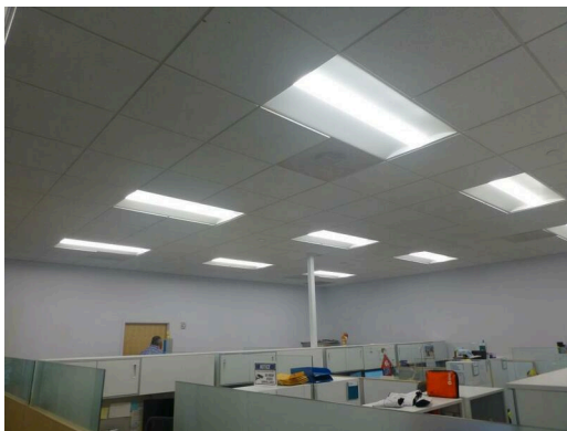
Office LED Lighting-Typical
