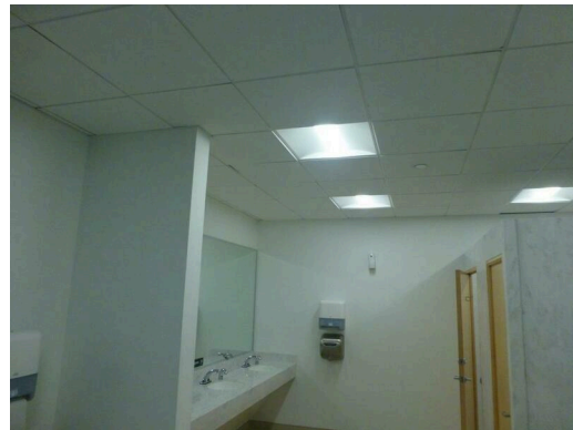
LED Lighting At Restroom
