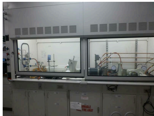
Typical LAB Hood with Sash Control
