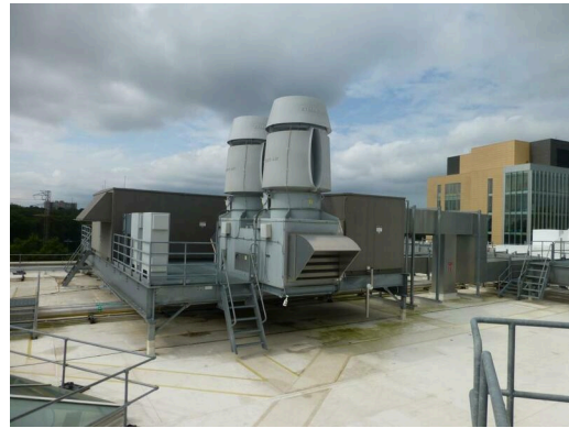
Strobic Fans and Rooftop
