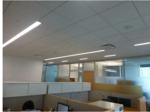
Corporate Office LED Lighting
