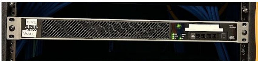
Novi Library's current firewall - Soon to be replaced
